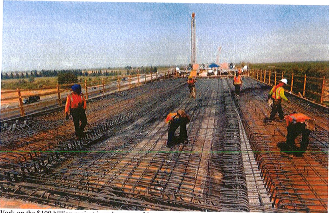
Work on the $100 billion project is under way at 21 construction sites in five counties, even though not all the necessary financing is in place. Workers installed reinforcing steel for a bridge across the San Joaquin River. Credit: Jim Wilson/The New York Times
